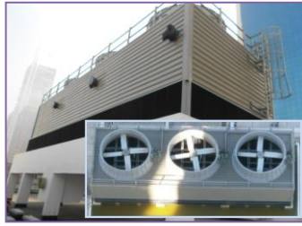
Cooling Tower (SPIG)
