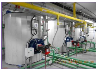
Gas Fired Boiler & Calorifier (PVI)
