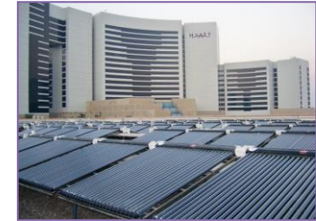
Thermal Solar System to Produce Hot Water (Tsinghua)
